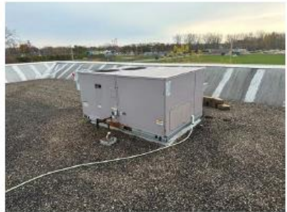
HVAC Roof-top Unit
